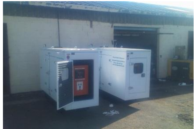
All Generators, Transformers UPS, and Inverters
