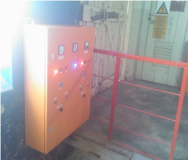
We design & Build control panels for pumps
